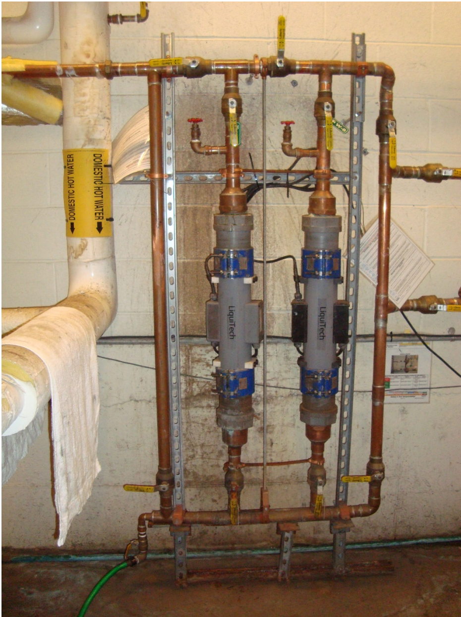
Figure 1 System installed at Maria Fareri Children's Hospital
