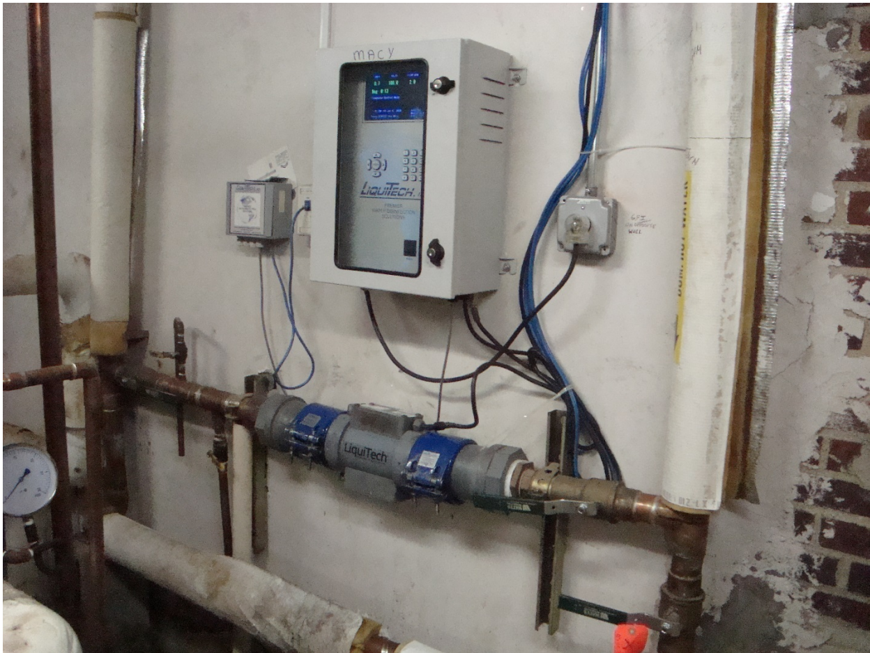
Figure 3 System installed at Macy Pavilion
